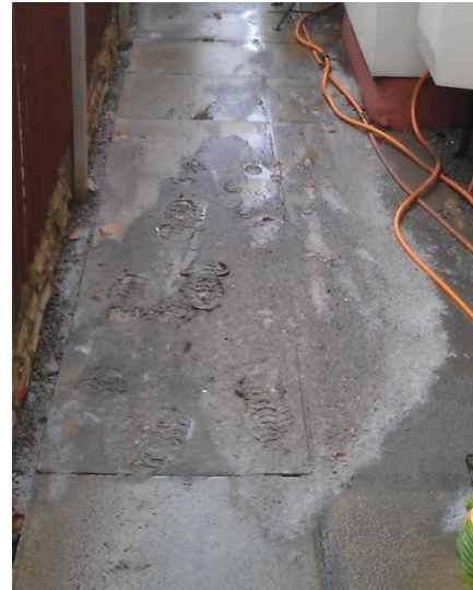
Figure 5: Foul debris residence side passage
