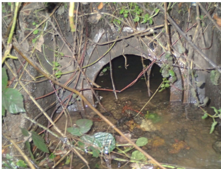
Figure 8: Outfall from Fouracres into Whinny Brook, taken 06/11/2012
